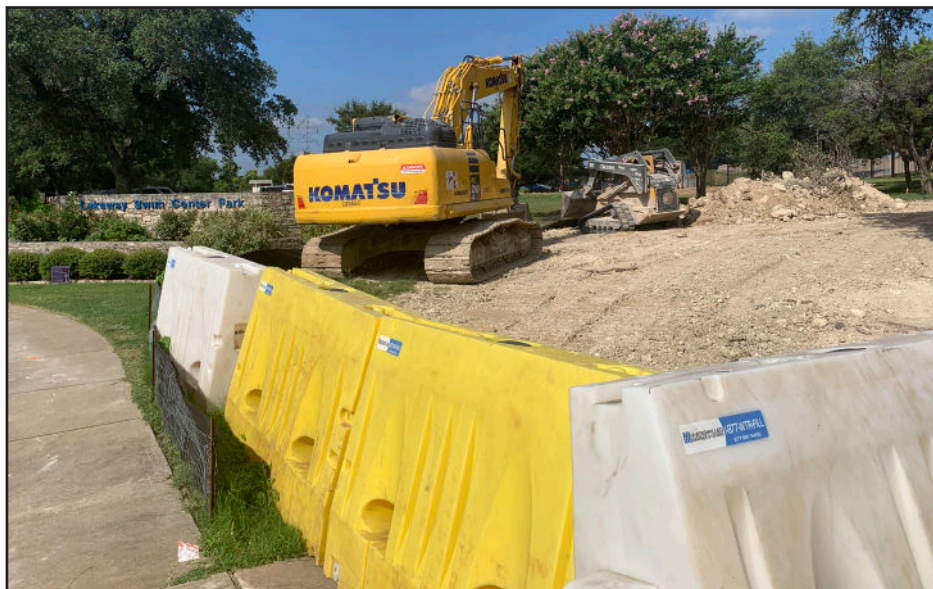
Our Out of District Wastewater (ODWW) Project, bringing public sewer access to the first 17 sections of Lakeway is fully underway. Last summer, heavy equipment could be seen at the Lakeway Swim Center as a sewer line was extended down the Lakeway Airpark airstrip, across Lakeway Blvd., to a wastewater treatment plant on Highlands Blvd.
